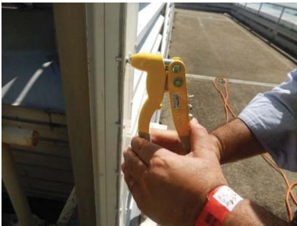
Fig. 10 Installation of new replacement rivets where 12-year-old rivets were extracted in March 2017
