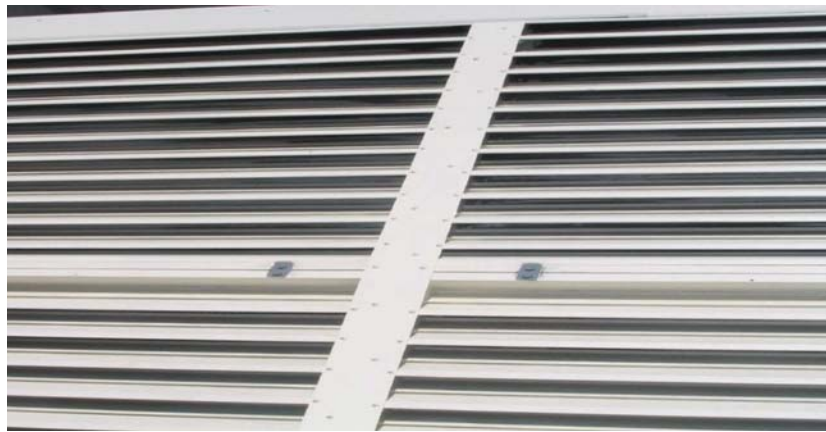
Fig. 5 Photo taken in June 2005, showing original Al 6061 flat strip riveted louver structure and two mullion sections connected and secured on Level 28 (identical to Level 29)
